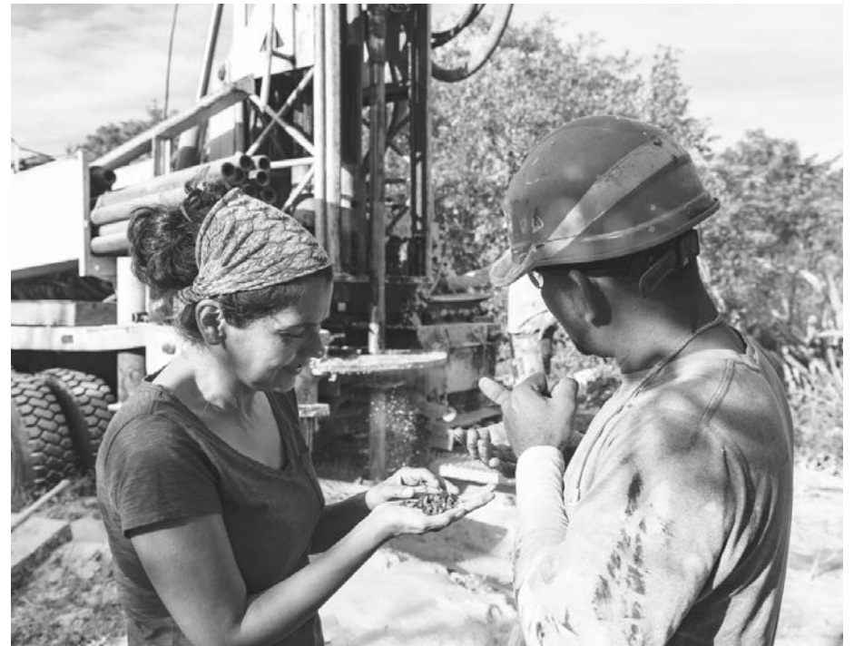
Teresa Camacho, one of Cross Catholic Outreach's international project officers, meets with workers operating a well-drilling rig to discuss the project's challenges.
